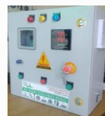
Control Panel / VFD
